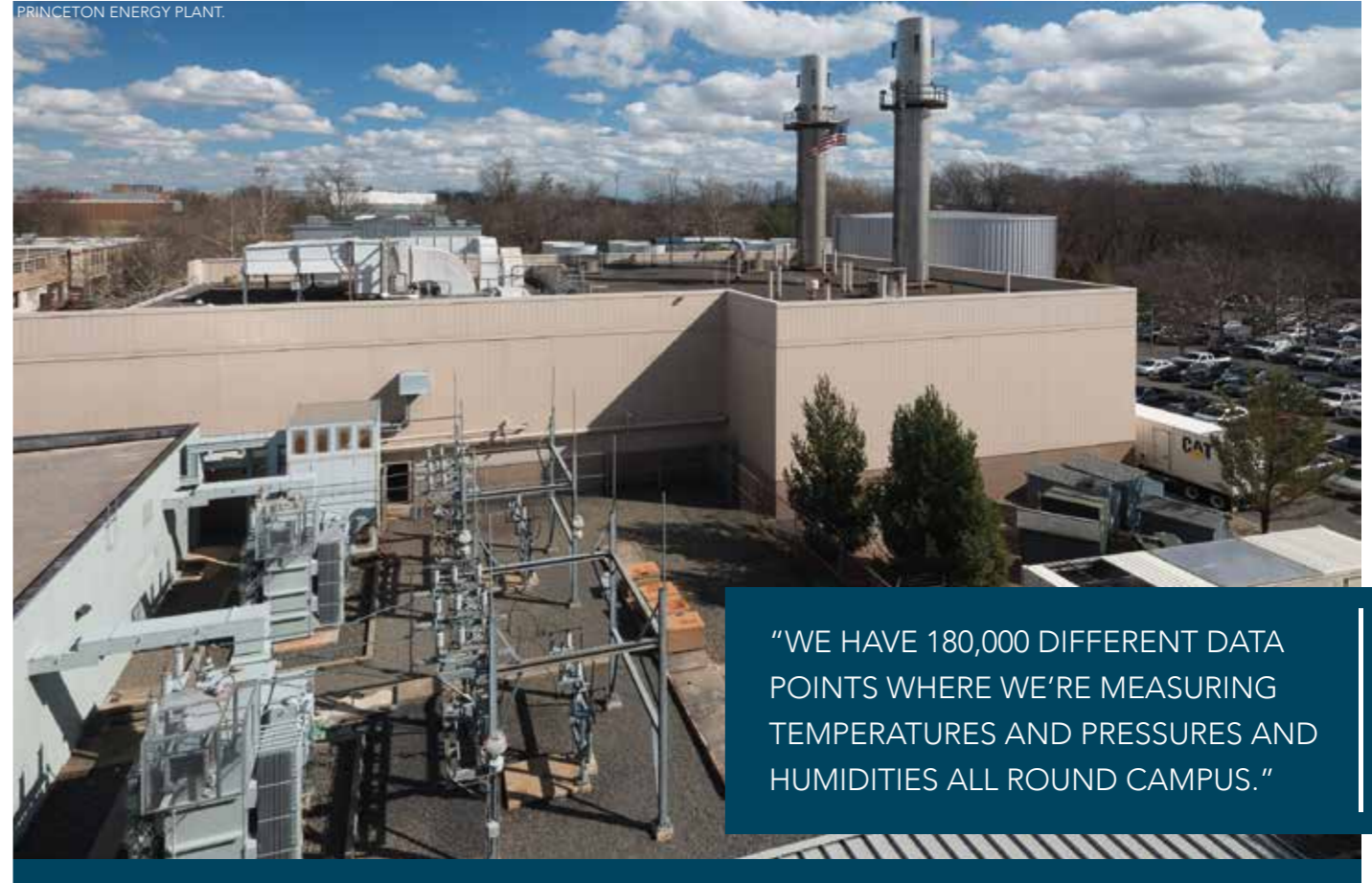
PRINCETON ENERGY PLANT.
